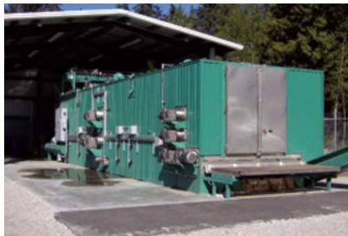
In-vessel high-rate composters quickly transform organic waste.
